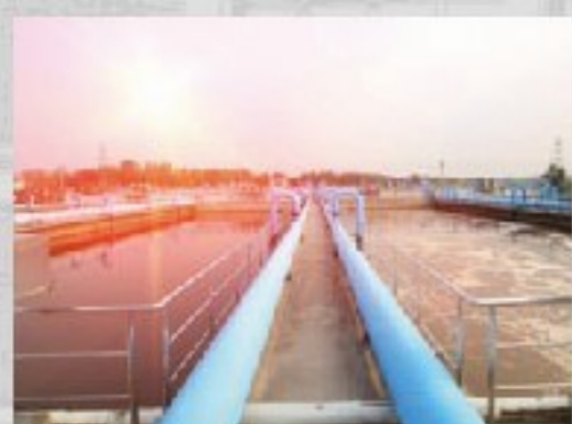
Water supply and drainage
